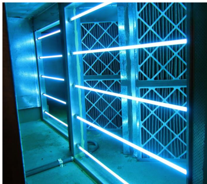
In duct/coil UVGI systems
