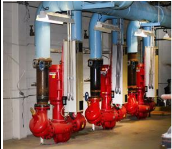
Chilled Water pumps & Condenser Pumps
